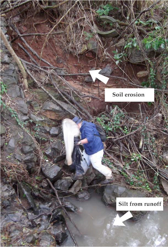
Stream bank erosion at upper pool below culvert
